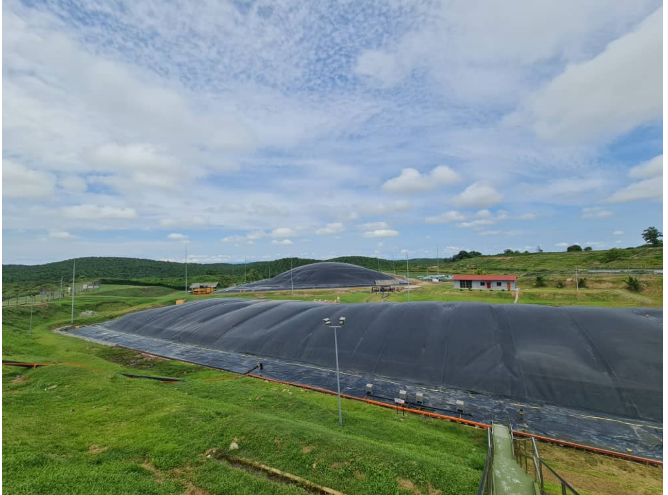
FGV's Triang biogas power plant
