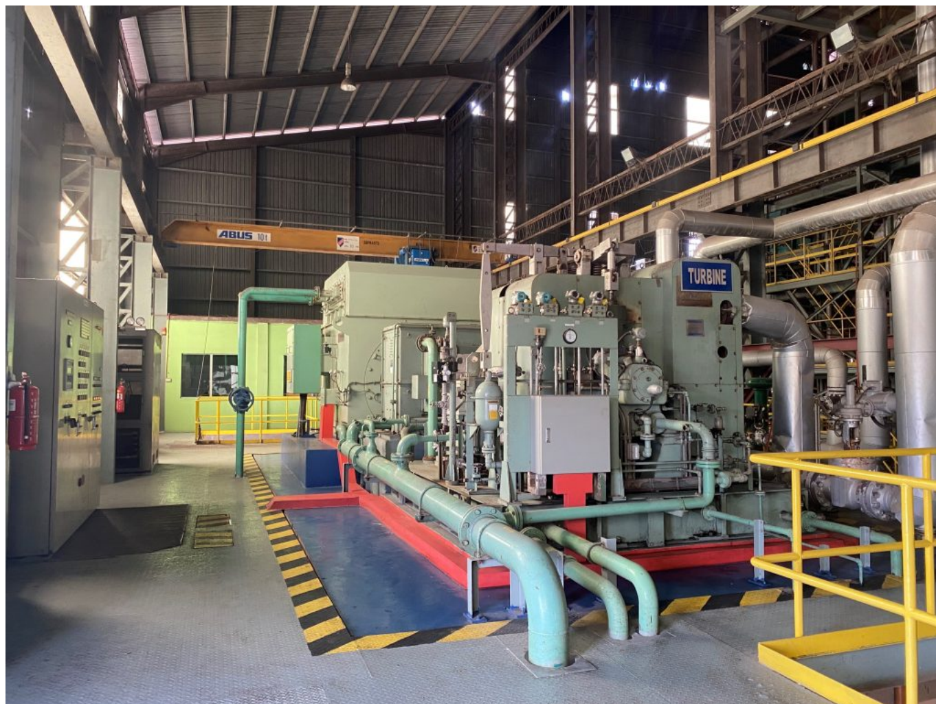
Generating electricity via steam turbine with a capacity up to 7.2MW
